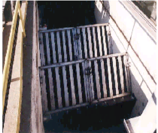
Internals of Monarch's API Concrete Basin shown with Separation Enhancements
